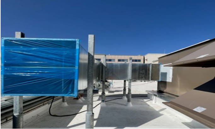
[From left] Exterior and interior views of construction progress at Los Robles Medical Center.
